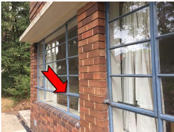
Photo 3. Exterior, southern elevation, window frames – asbestos-containing mastic sealant.
