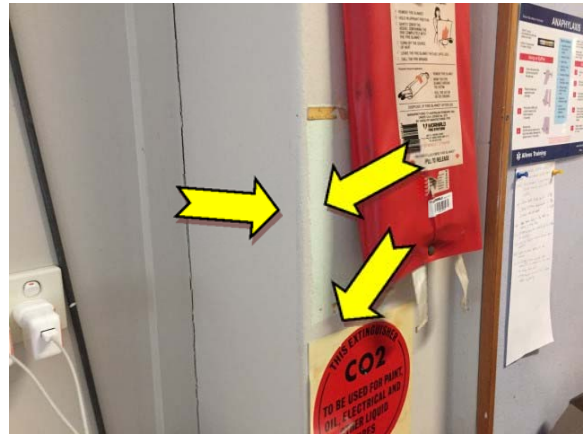
Photo 10. Interior, kitchen, walls – suspected lead-containing grey upper paint systems and green lower paint systems.
