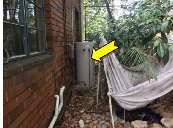
Photo 8. Exterior, south-west elevation, hot water heater – suspected internal SMF insulation.
