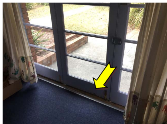
Photo 12. Interior, door and door frames – lead-containing yellow lower paint systems.
