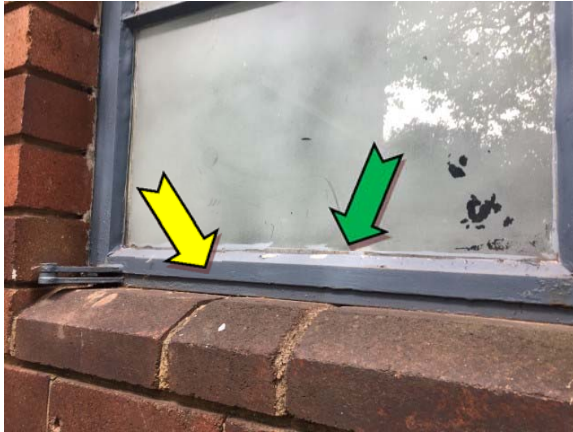
Photo 1. Exterior, north-eastern elevation, window frames – non asbestos-containing window caulking and suspected lead-containing blue upper paint system.
