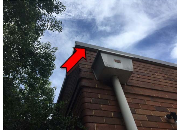
Photo 2. Exterior, throughout, eaves – suspected asbestos-containing fibre cement sheeting.
