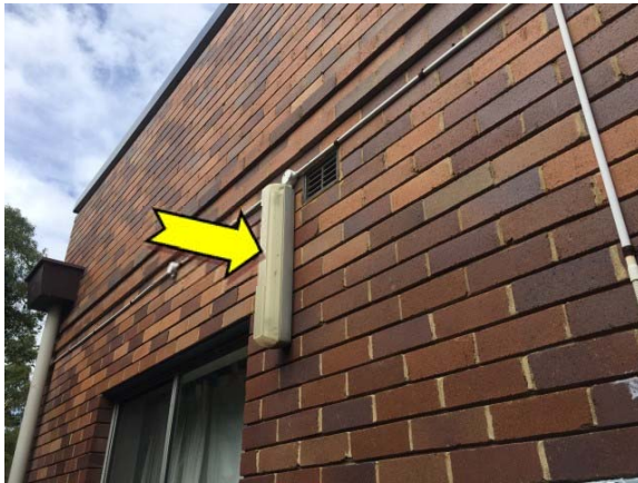
Photo 9. Exterior, single tube fluorescent light fittings – suspected PCB-containing capacitor.
